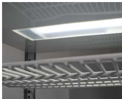
Internal lighting in the ceiling
